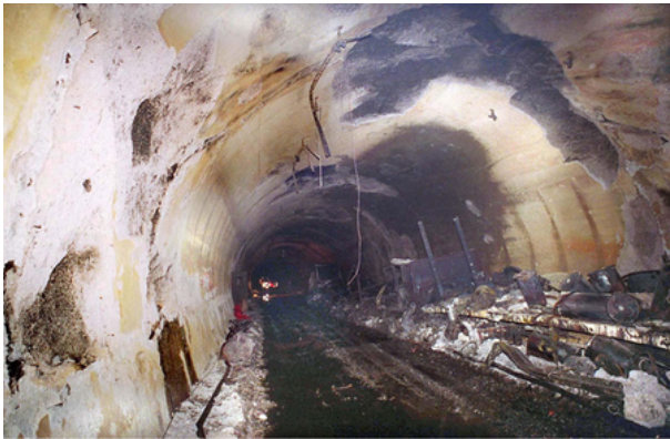
Fire incident in the Mont Blanc tunnel in 1999 Source: Kaundinya 2007
